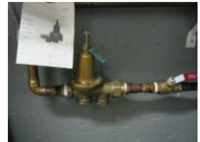
Pressure Regulating Valve (PRV)
